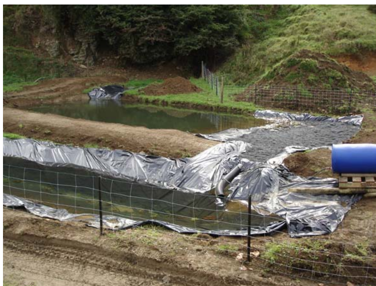
Photograph 5: Temporary Spring Flow Treatment System
