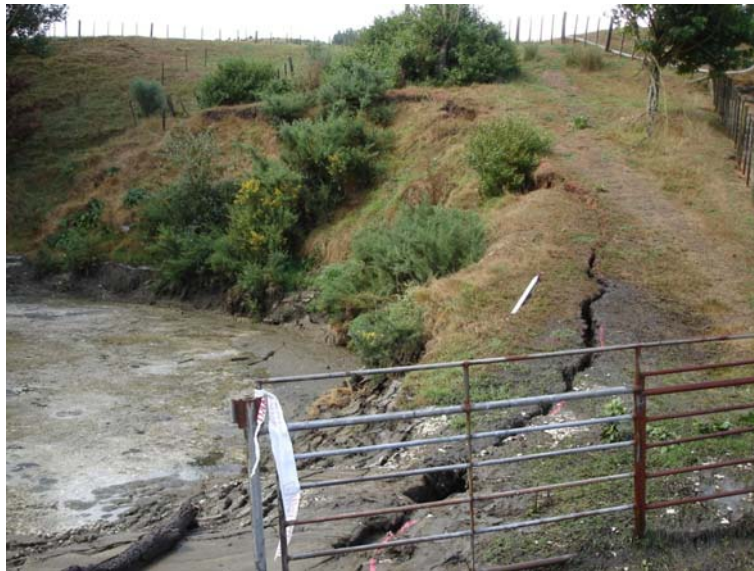
Photograph 3: Fissure Formation near the Sinkhole
